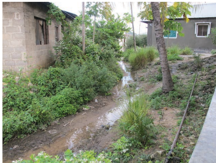
Picture: Leakage from the pipe creating a stream at eastern zones in Makadara
