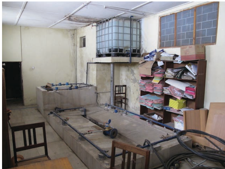
Picture: Meter inspection yard
